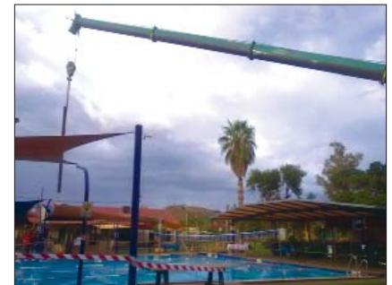
A crane lowers the support beams for the new 50 meter pool shade sails
