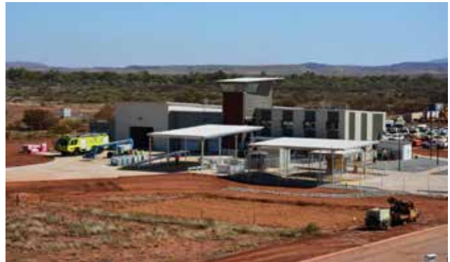
Final site handover is scheduled for July 2014, and the station to be operational by the end of August 2014.
