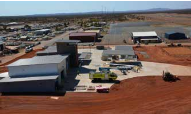
All major construction to the ARFF (Airport Rescue and Fire Fighting Station) has been complete.
